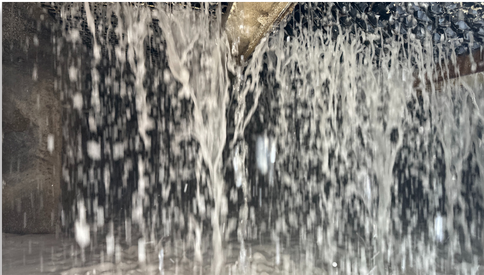
RYDLYME circulating through a cooling tower via the tower's pump
