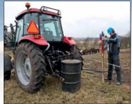
The HYCON Post Driver is very easy to use onboard a tractor in the field.
